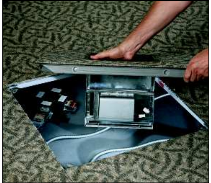
This photo displays the major HVAC, power and carpeting components that make integrated access-floors worth exploring for most any information-technology facility, especially call centers.
